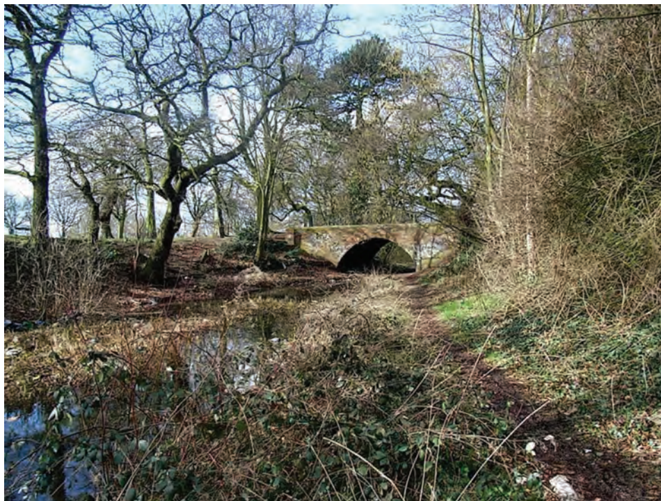
Accommodation bridge over the Lapal Canal in Selly Oak Park. This is an original bridge that was provided for pedestrians (and animals) when the canal was built in 1798. It is now believed to be one of Birmingham's two oldest surviving canal bridges although there are railings instead of the original parapet. Restoration of the canal is not permitted at present because of drainage issues. These will be resolved with the development of Battery Park where the Lapal Canal will connect with the Worcester and Birmingham Canal.
